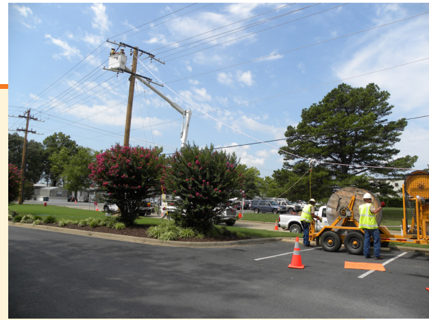
Electric Department crews had several projects in 2014 reconductoring circuits. Reconductoring upgrades the current carrying capacity of distribution line circuits.
