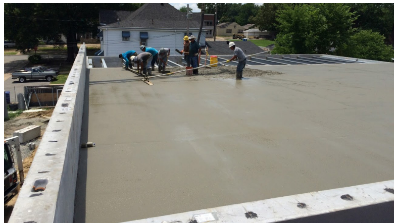
Conway Corporation's new data center is constructed to withstand winds up to 250 miles per hour.
