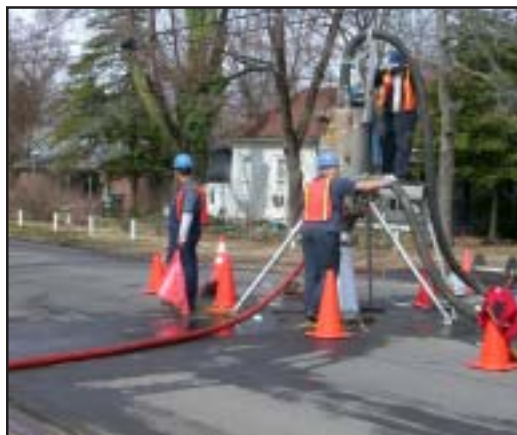
A CIPP (Cured-in-place-pipe) was used to repair approximately 1,500 feet of the sewer main on College Ave.
