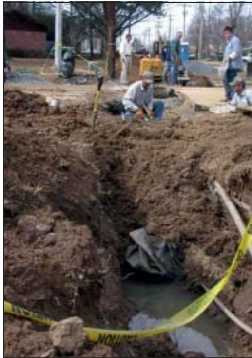
Employees of contractor Paladino-Nash Construction work to replace a water line along College Avenue.
